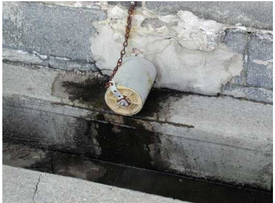
Figure 9. Drain plugs must be sealed to keep out flies and especially rodents.
